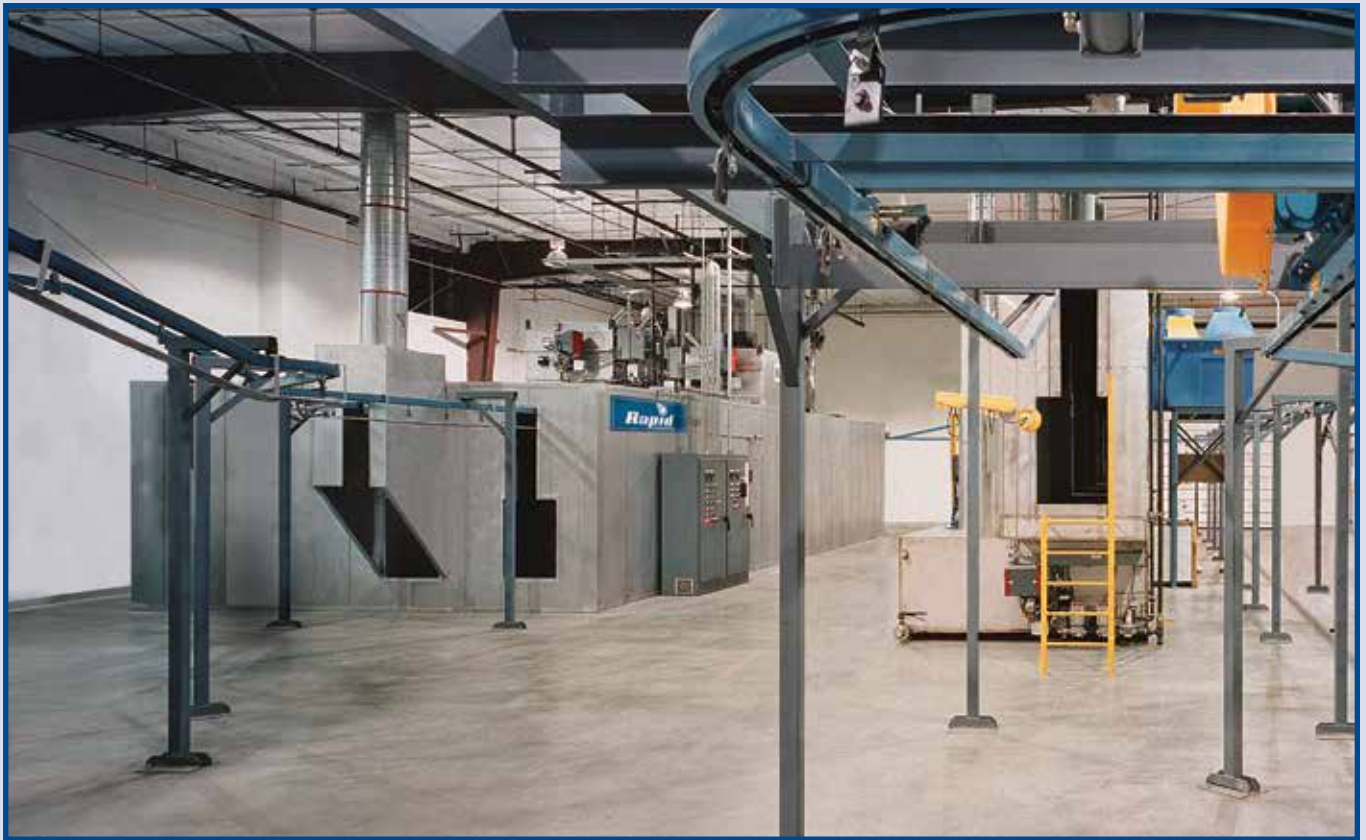
A typical RAPID® finishing system with five-stage washer, dry-off oven, cure oven, conveyor and controls.
